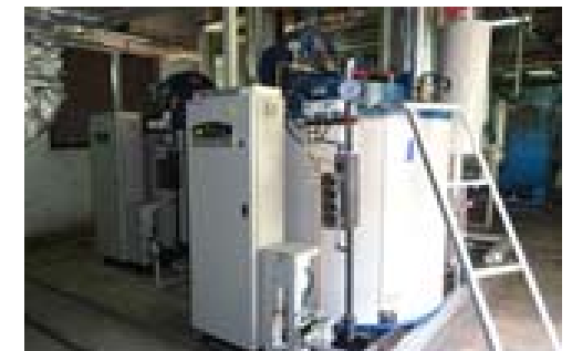
【Low carbon hotel by development of BEMS】 (Viet Nam) 605tCO 2 /y. Start operation: Jan. 2017
