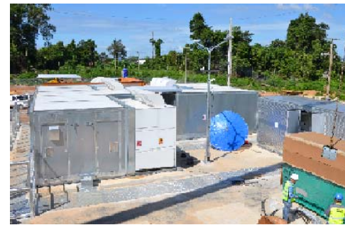
【Energy-efficient data center】 (Laos) 1,074tCO 2 /y. Start operation Jan. 2017
