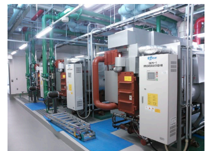
(c) Absorption Chiller (Genelink)
