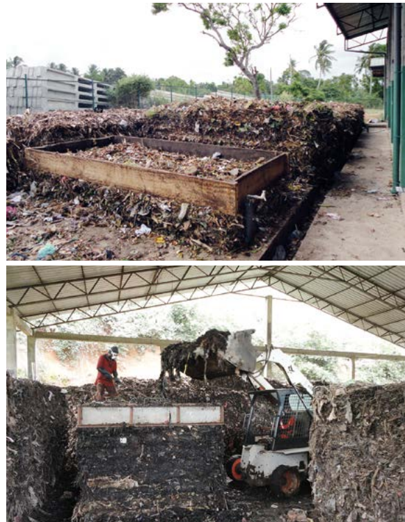
Fig. 35 Piling up composting feedstock using wooden frame and skid steer loader (Karunarathna, 2020)
